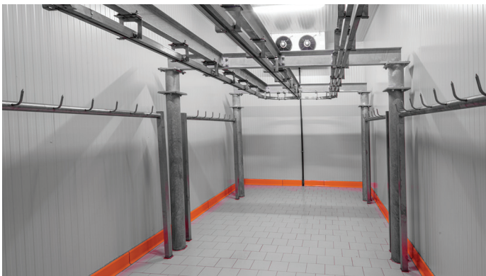
Cold Room and Storage
